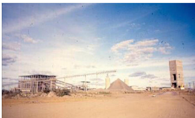
FIGURE 10 - Construction of concentration and underground mine facilities in the early days at Caraíba. A looking-to-the-East view of the secondary crusher (to the left) and the tower of the main shaft (right), all still under construction in the early days of 1978, coevally with the first days of mine operation in the open pit. The stockpile seen in the middle grew up with the first loads of ore exploited from the open pit (bench 440 m), which was used for testing the primary crusher (further left, outside the picture, from where departs the inclined conveyor belt). The underground mine was not contributing with ore, at that time, yet.
