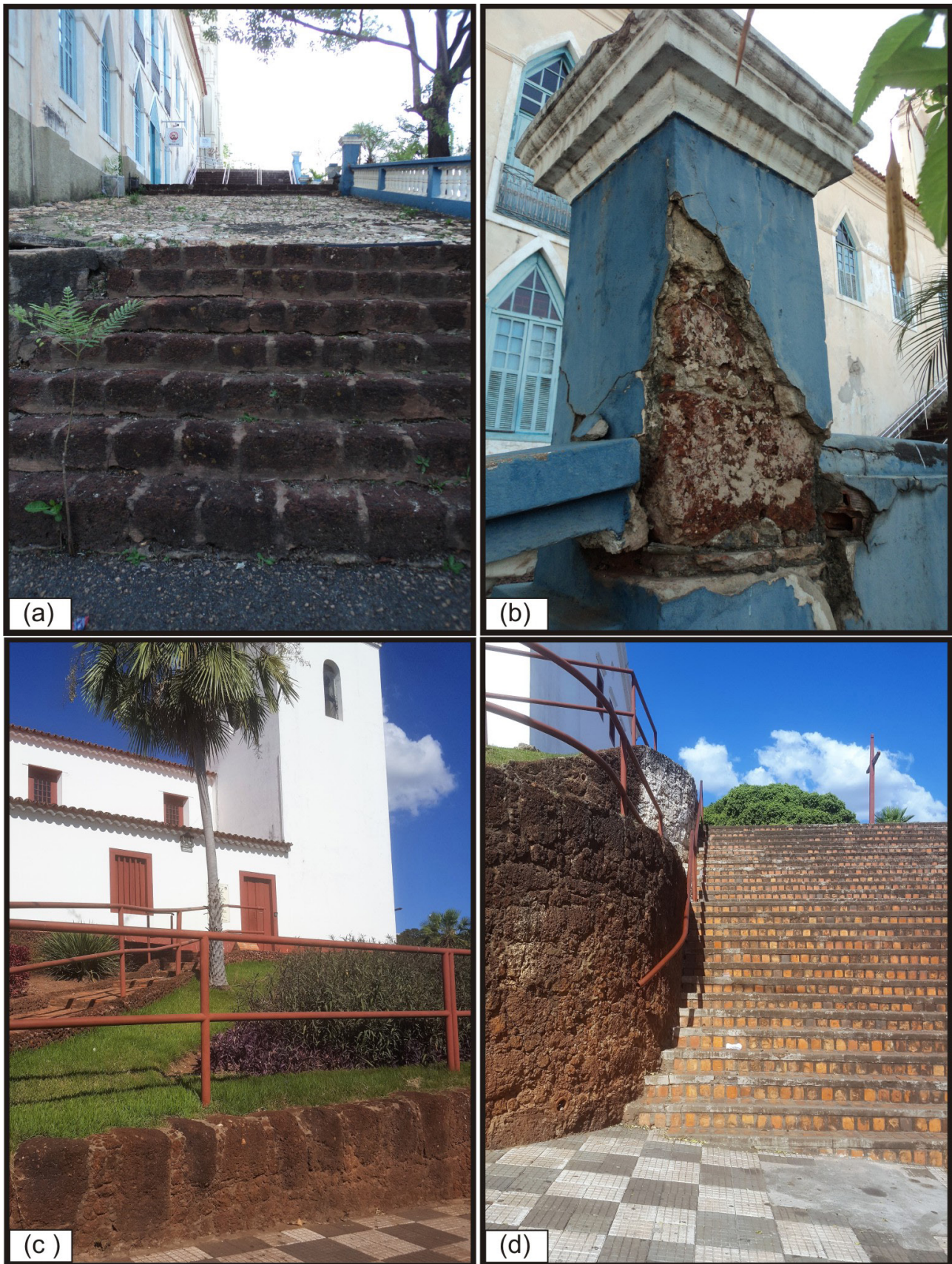
FIGURE 5. (a) and (b). Side stairway and pillar of the old wall of the Church of Nossa Senhora do Bom Despacho; (c) and (d) Protective wall and sideway/stairway, made with ironstone, of the Church of Nossa Senhora do Rosário e São Benedito, Av. Coronel Escolástico (Source: Ana Costa, 2020).
