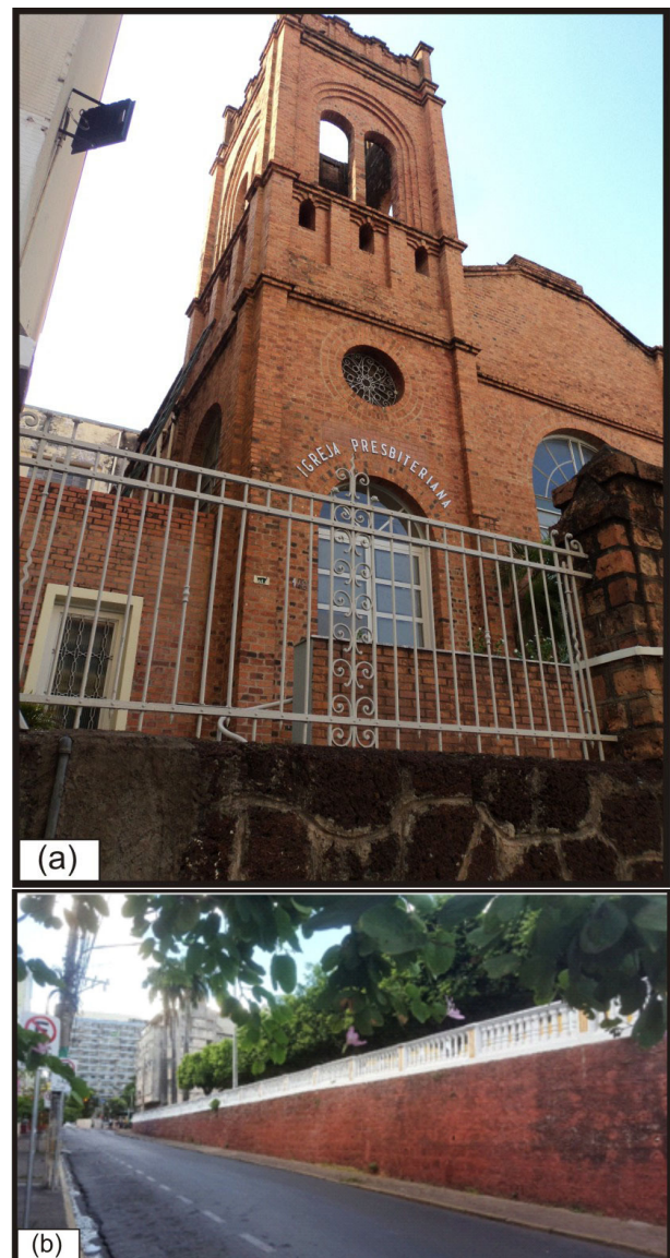
FIGURE 2. (a) Detail of exposed bricks and ironstone wall of the Presbyterian Church of Cuiabá, MT; (b) Back wall of the Instruction Palace, made with ironstone and currently covered with paint (Source: Ana Costa, 2020).
